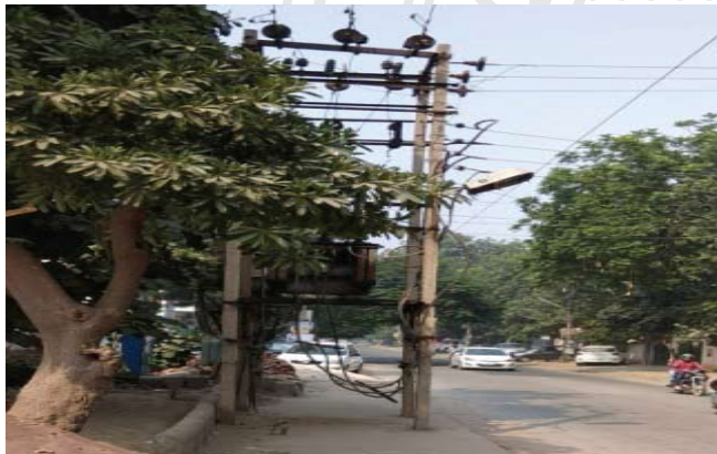
Figure 23: Dangerous Obstruction on the Footpath
